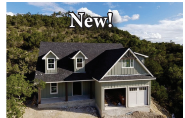
1185 Soaring Eagle MLS 7997675 Under construction. 4/2.5 two-story modern farmhouse style home. $685,000 Jim Donaldson
